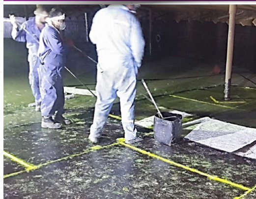
▲ The implementation of composite coatings on the floor of a corroded tank
